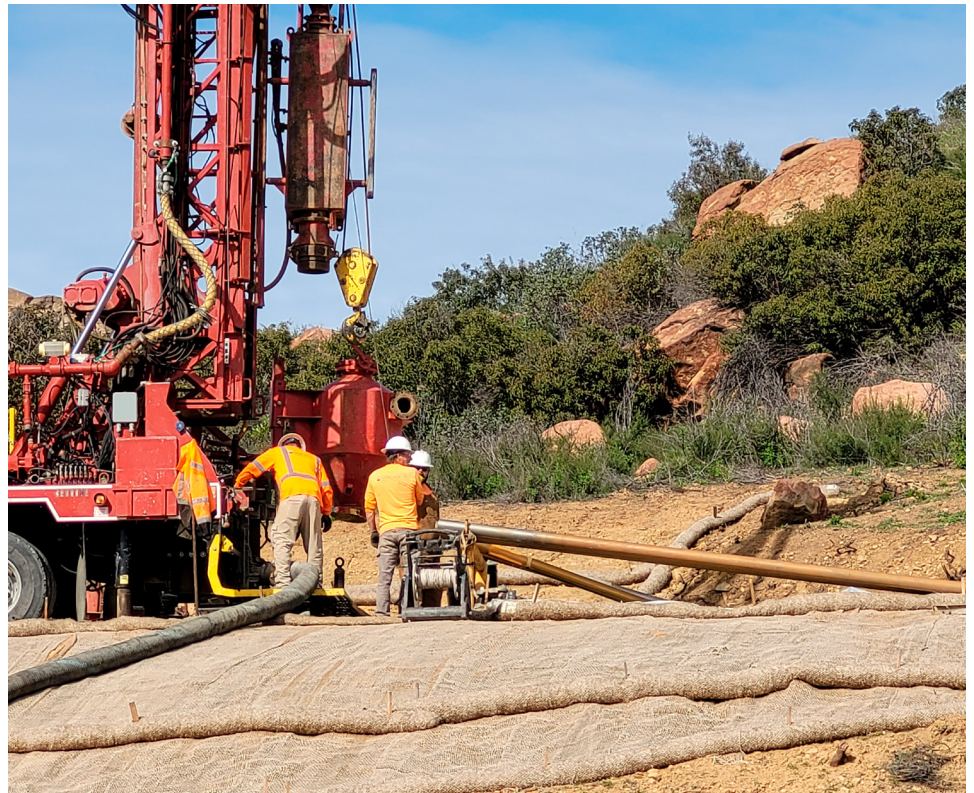
Crew installs bedrock vapor extraction well near the former Component Test Laboratory III.
