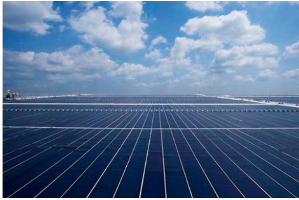
The 10-acre solar system at the Boeing North Charleston, South Carolina, facilities continues to be one of the largest thin-film solar installations in the United States. (Boeing photo)
