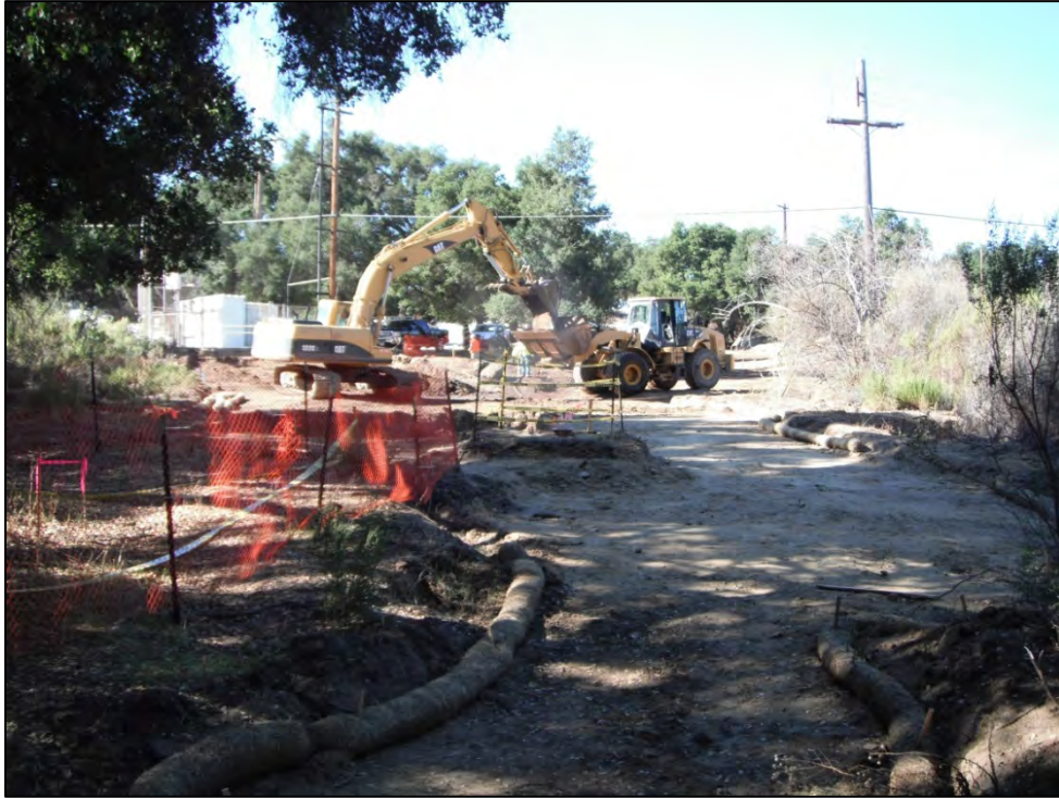
View of ISRA area AP/STP-1C-1 (eastern portion) during additional soil removal activities (10/31/2012, looking west).
