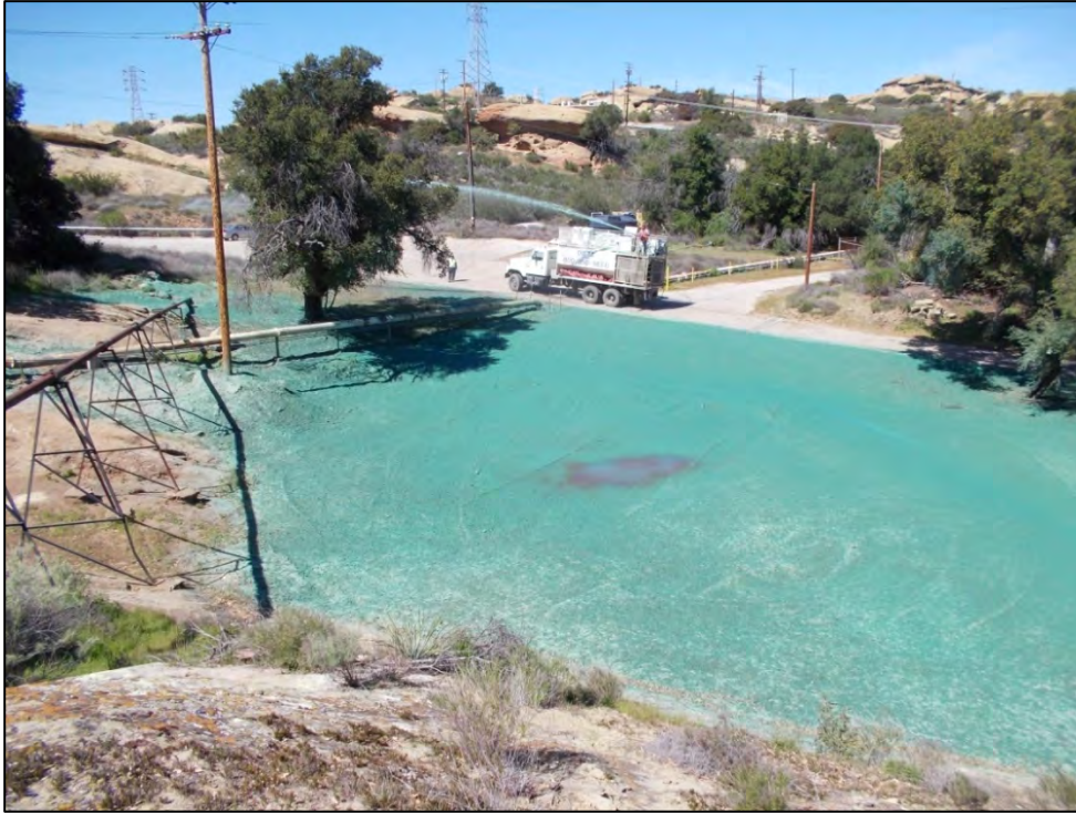
View of ISRA area AP/STP-1B (western portion) after hydroseed application (3/8/2013, looking northwest).
