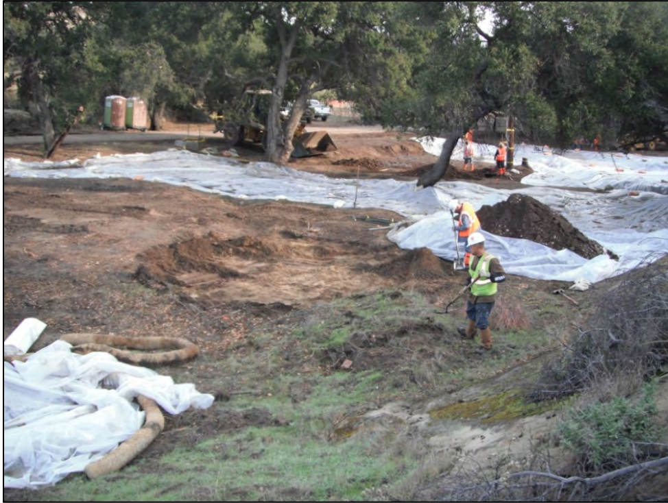
View of ISRA area AP/STP-1B during excavation of central and eastern portion (11/23/2011, looking northeast). Excavation area was covered during rain events.
