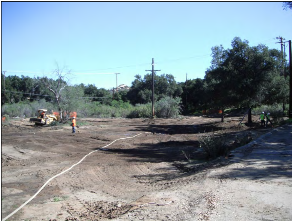
View of ISRA area AP/STP-1C-1 (near southwest corner) during contouring (3/1/2013, looking northeast).
