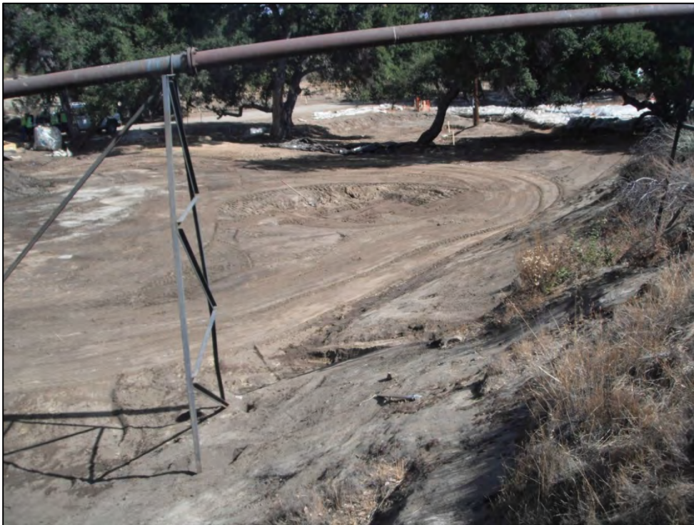
View of ISRA area AP/STP-1B from southwest corner after excavation (10/5/2012, looking northeast).
