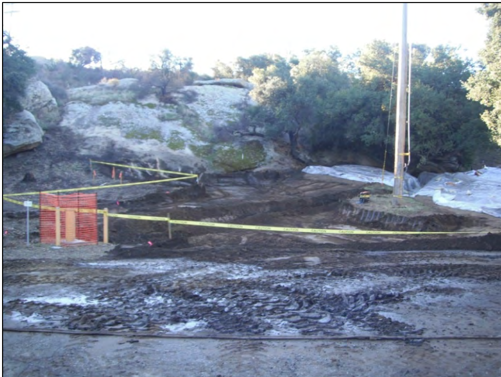
View of ISRA area AP/STP-1B during excavation of eastern portion (11/17/2011, looking south). Plastic tarps placed over excavation area during rain events.
