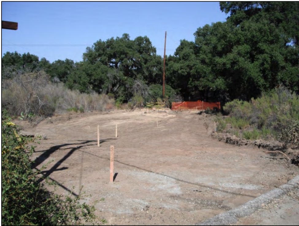
View of ISRA area AP/STP-1C-1 (near southeast corner) after excavation activities (9/26/2012, looking northeast).
