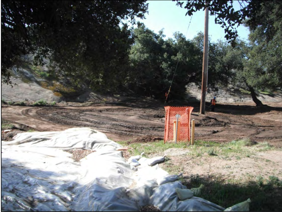
View of ISRA area AP/STP-1B during soil contouring of eastern portion prior to hydroseeding (3/5/2013, looking south-southwest).
