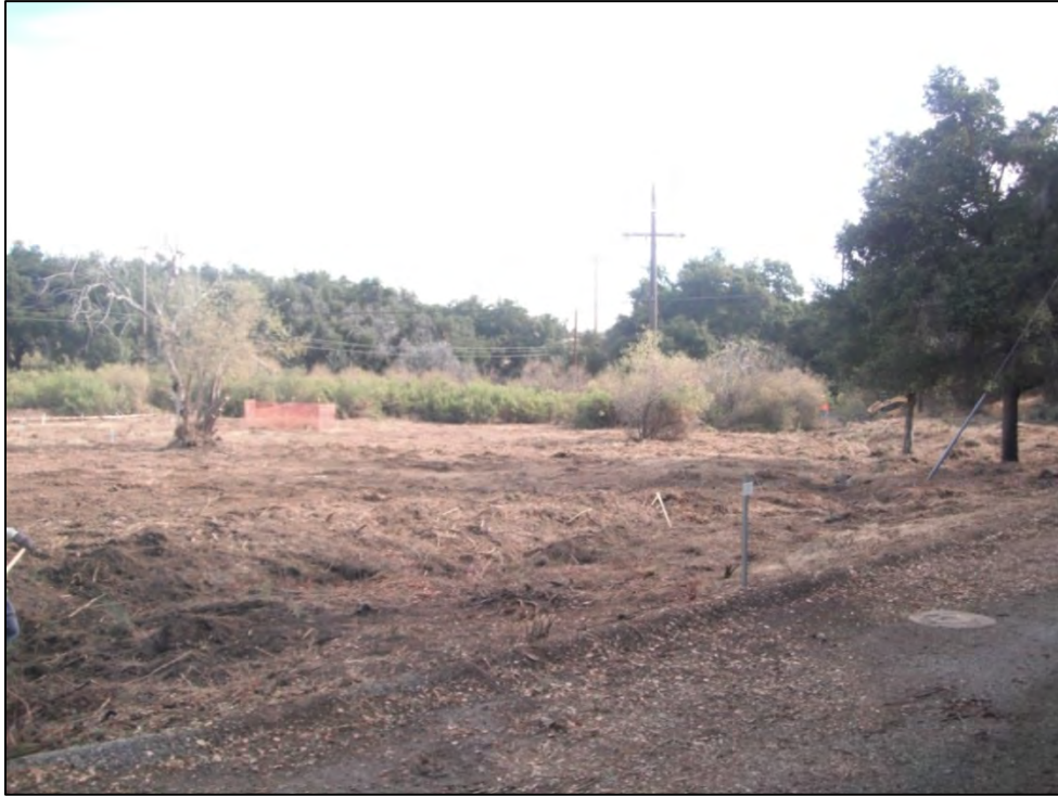
View of ISRA area AP/STP-1C-1 (near southwest corner) after vegetation clearance and prior to excavation (11/22/2011, looking northeast).
