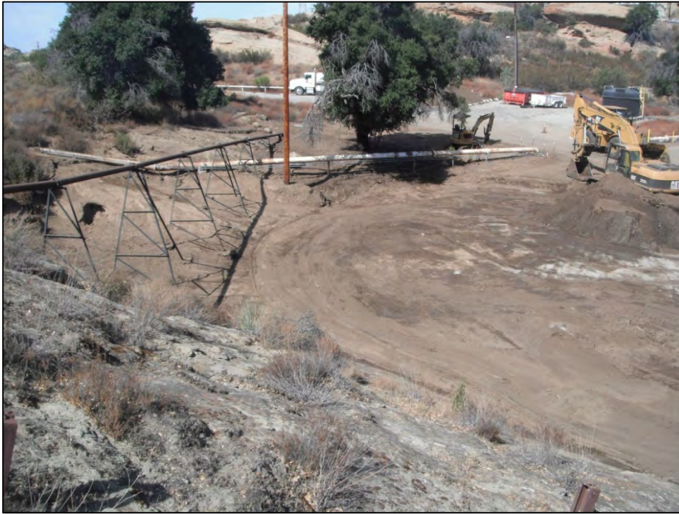
View of ISRA area AP/STP-1B during excavation of western portion (10/5/2012, looking northwest).
