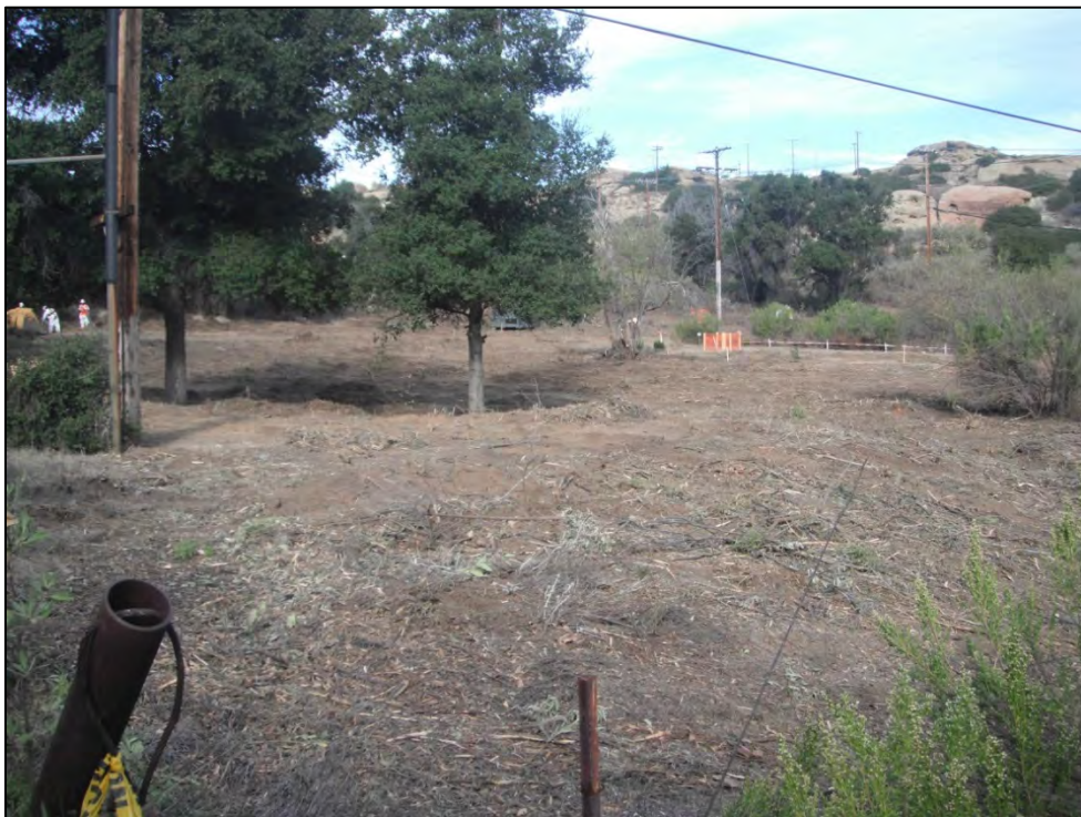
View of ISRA area AP/STP-1C-1 (near southeast corner) after vegetation clearance and prior to excavation (11/22/2011, looking northwest).
