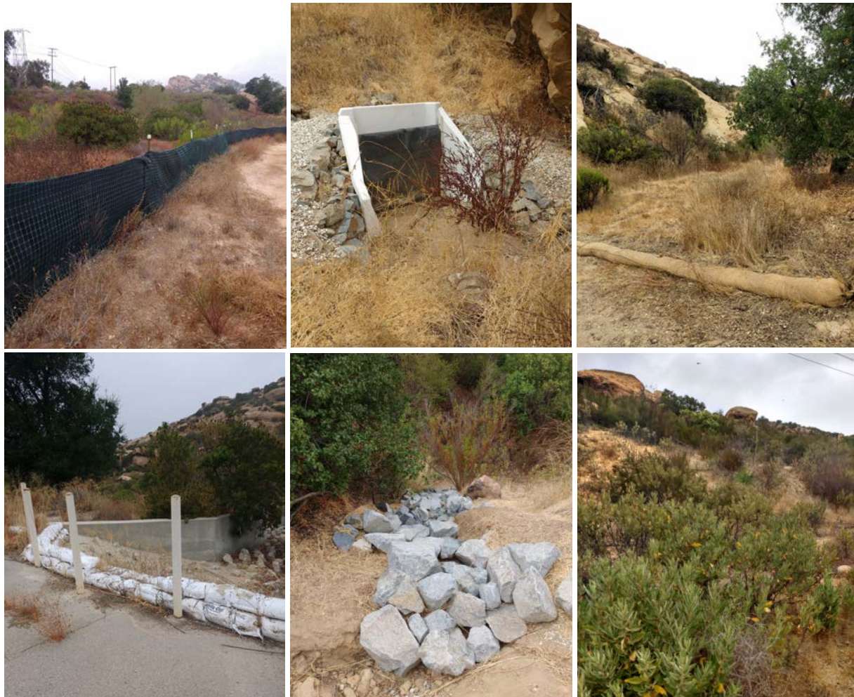
Figure 3. Selection of Existing BMPs at the Former Shooting Range Area (Top row: Silt fence, culvert modification media filter, and fiber rolls; Bottom row: Sand bag berm, rip-rap, and vegetation)
