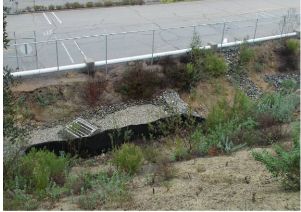
2012: B-1 Sedimentation Basin and Media Filter
