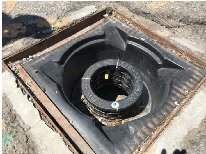
Figure 19. Administration Area Inlet Filter: Potential for Short-Circuiting around the Lip
