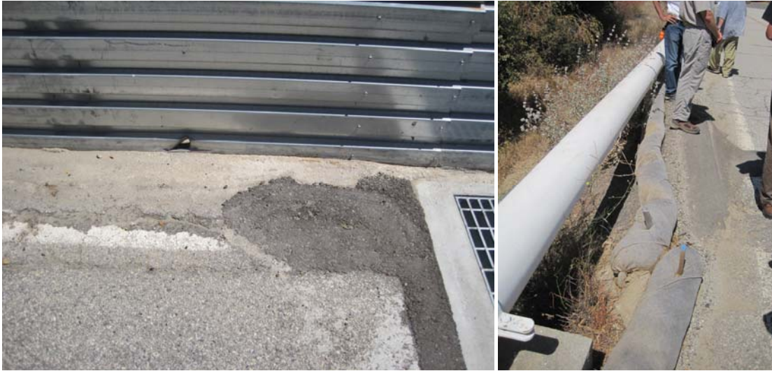
Figure 18. CM-3 Road Runoff Inlet: Sheet Metal Wall (left) and Fiber Rolls (right)
