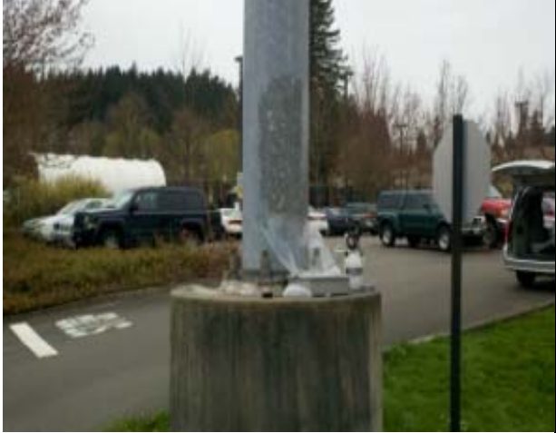
Utility pole, galvanized; NB Kitsap
