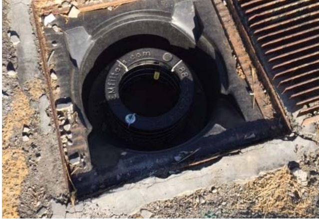
2017: Administration Area Inlet Filters (Filter Basket)
