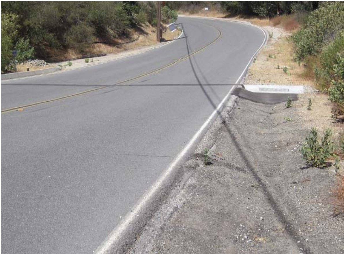
Figure 10. CM-1 Road Runoff Diversion
