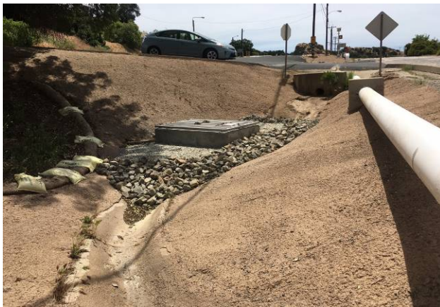
2017: Upper Parking Lot Media Filter
