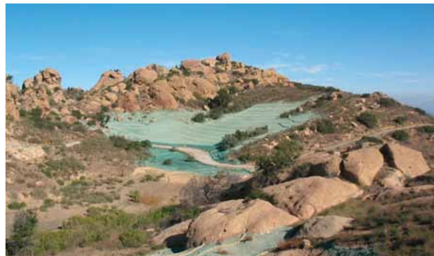
After soil was removed, excavated areas were back filled, recontoured and hydroseeded.
