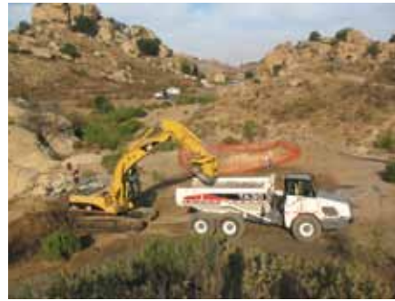
Water was used as a dust control measure when soil was removed from the outfall and loaded into transportation trucks.
