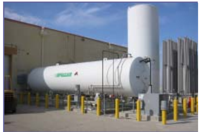
LCO 2 storage tank outside the IMF
