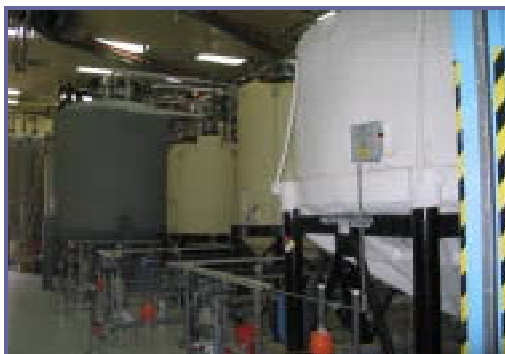
BHP mix room inside the IMF
