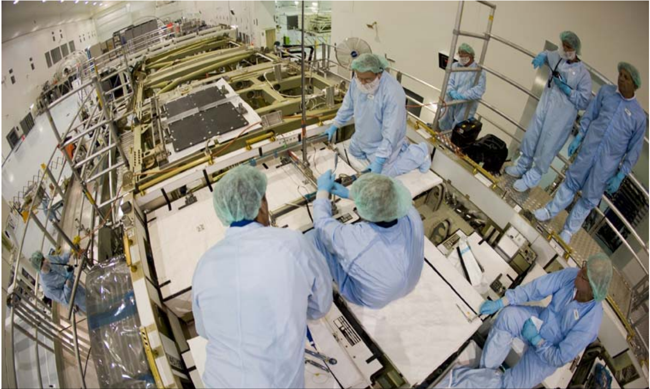
Under Boeing’s Checkout, Assembly and Payload Processing Services (CAPPS) contract, Boeing technicians are installing new batteries on the Starboard 6 truss. The batteries had to be replaced because they had exceeded their life limits as a result of the delays caused by the Space Shuttle Columbia accident. The batteries were replaced in the summer of 2009. (Indyne photo by Dave Brinko)
