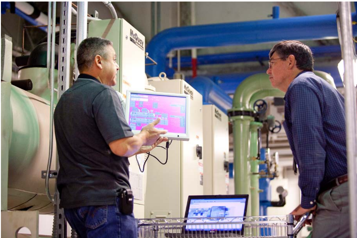
Rick Rivas, Boeing Site Services manager and Bill Richard, Boeing Site Services director, check a control panel for the Houston site's state of the art heating, ventilation, and air conditioning system. The system has helped the site save $250,000 since its installation.
