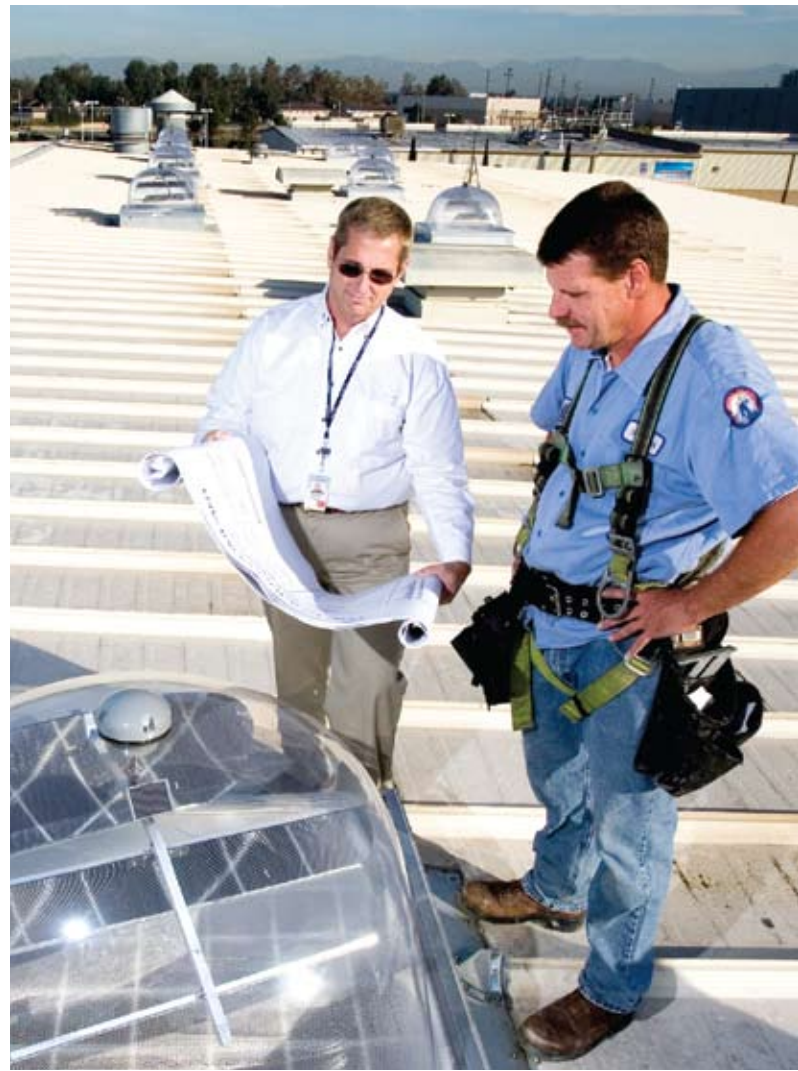
Steve Evans (left), utilities focal for Boeing's Site Services, consults with Lavey Roofing's Shannon Booth on the installation of solar-tracking skylights atop a 20,000-square-foot (1,858 square meters) office building in Huntington Beach, Calif. Solar-tracking skylights help reduce energy bills and Boeing's overall carbon footprint.
