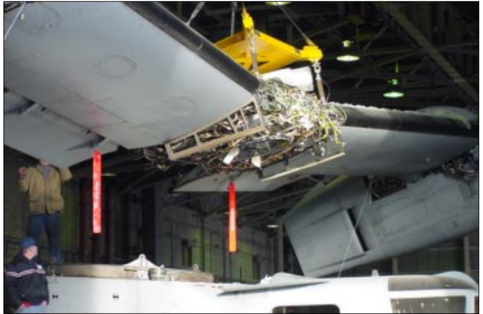
A 40-ton crane removes the wing of Aircraft Maintenance Trainer No. 11. The wing has been trucked to Ft. Worth, Texas, where it will be used to help test the tooling designed for the Block A modification.
