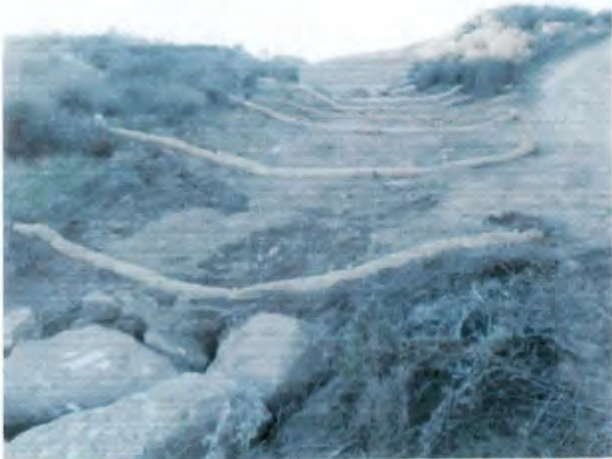
Re-contoured excavation and BMPs at ISRA area CTLI-1B. Hydroseeded and containerized plants to be installed.
