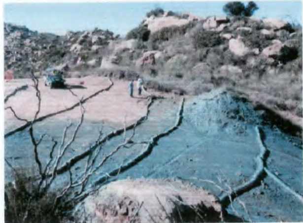
Hydroseeding ISRA area CTLI-1A following re-contouring and BMP installation. Containerized plants to be installed.
