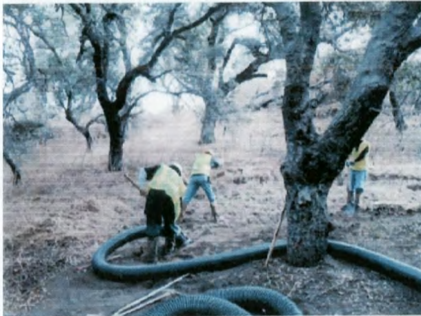
Excavation activities at ISRA area AP/STP-1F, loosening soils with hand tools under oak trees.
