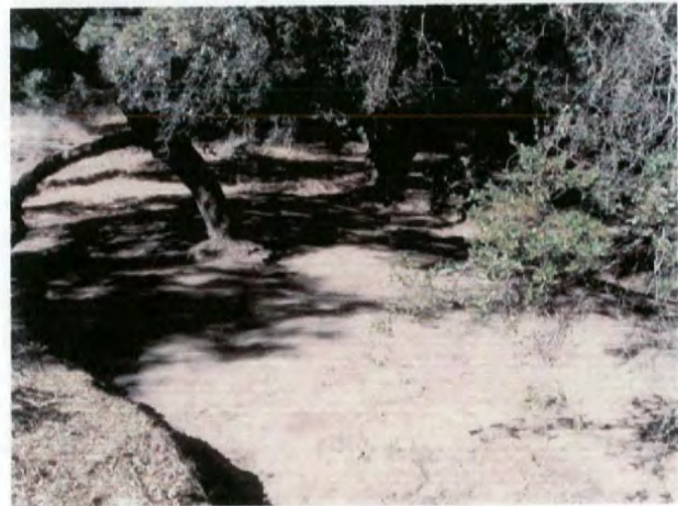
Completed excavation at ISRA area AP/STP-1F; excavation depth was limited to 1 foot under oak trees.
