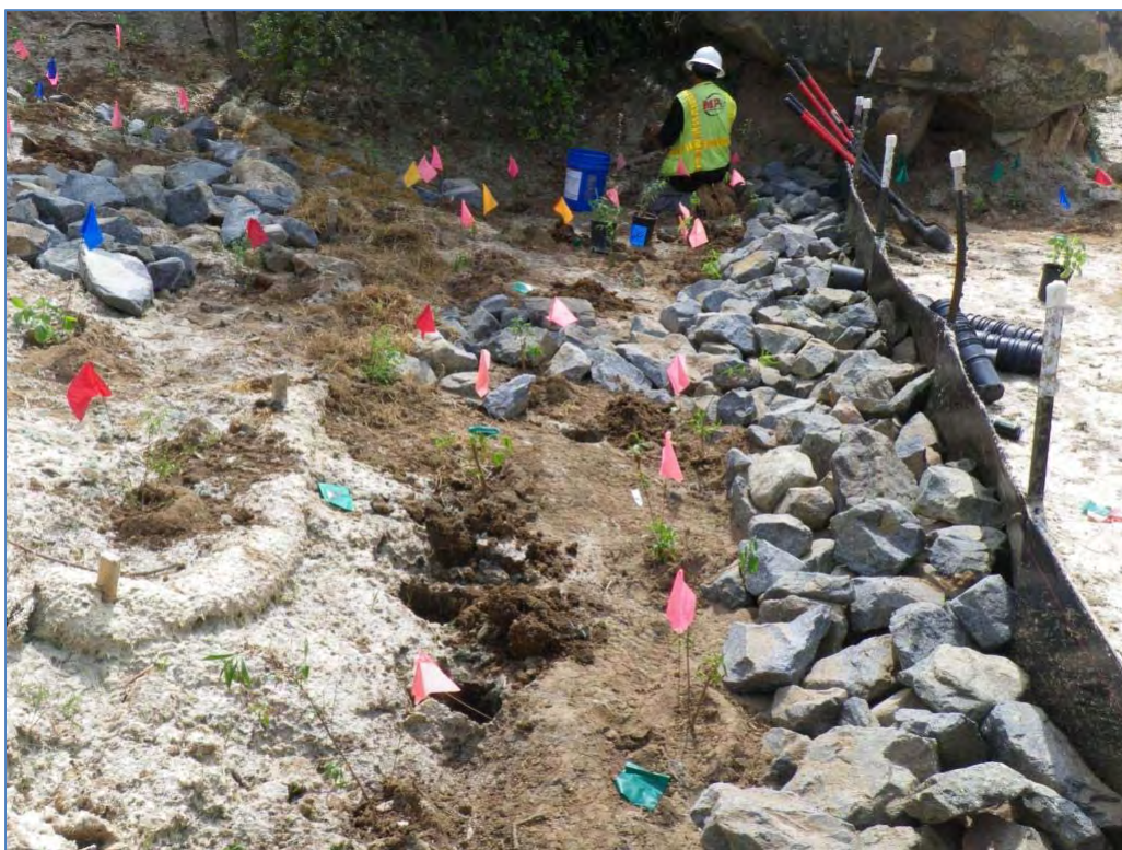
ISRA area B1-1A after restoration, during installation of containerized plants (3/17/2011, looking southwest). Pin flags mark the locations of installed plants.
