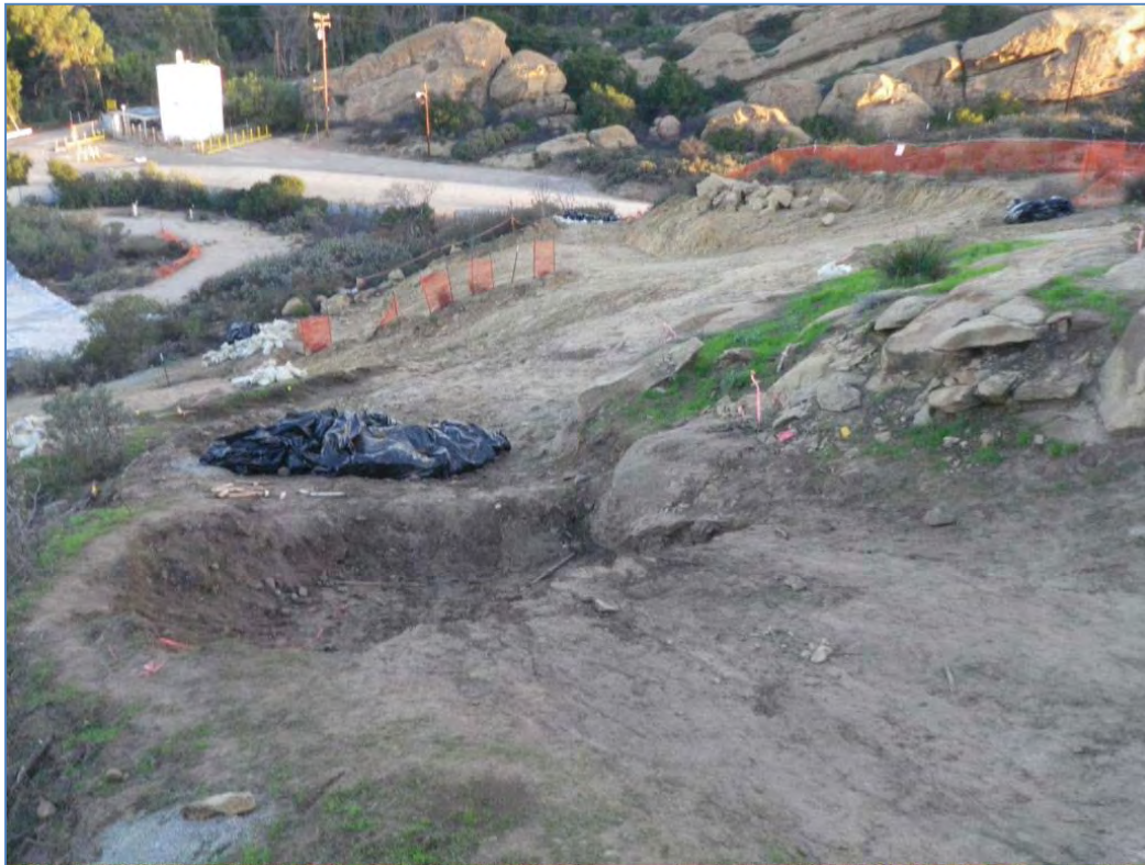
ISRA area B1-1C in foreground and ISRA area B1-1B in background after excavation (10/29/2010, looking north).
