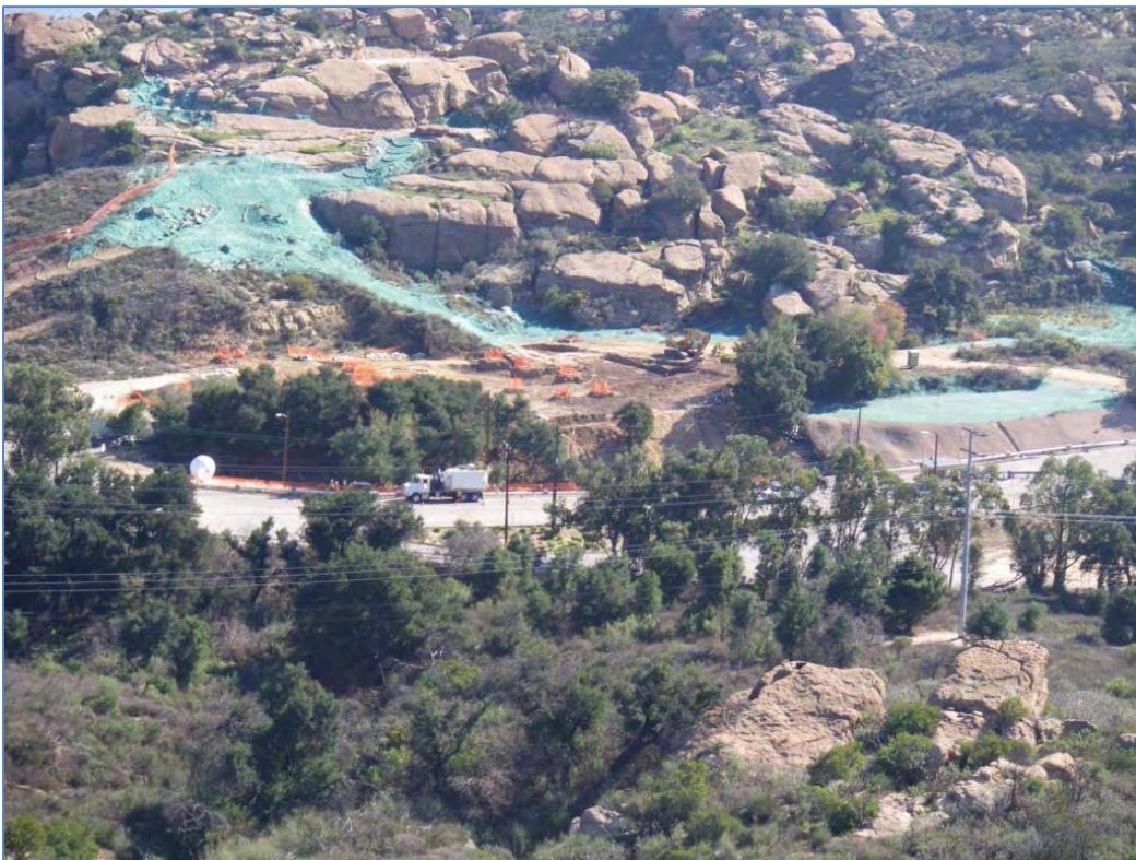
ISRA areas B1-1 and B1-2 after restoration at ISRA area B1-1, and during excavation at ISRA area B1-2 (11/16/2010, looking south). Blue-green hydroseed mulch is visible.
