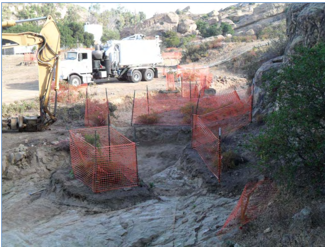
ISRA area B1-1A after excavation (10/1/2010, looking northeast). Bedrock exposed in excavation floor is visible in the foreground. Orange fencing around Santa Susana tar plants.
