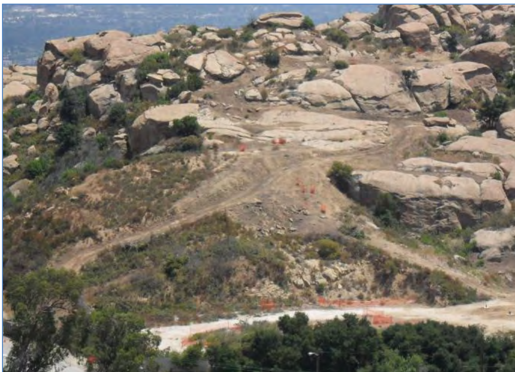
ISRA area B1-1B after vegetation clearance, prior to excavation (7/16/2010, looking south). Orange fencing around Santa Susana tar plants.
