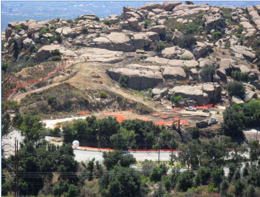
ISRA areas B1-1 and B1-2 after excavation at ISRA area B1-1, and during excavation at ISRA area B1-2 (8/23/2010, looking south).
