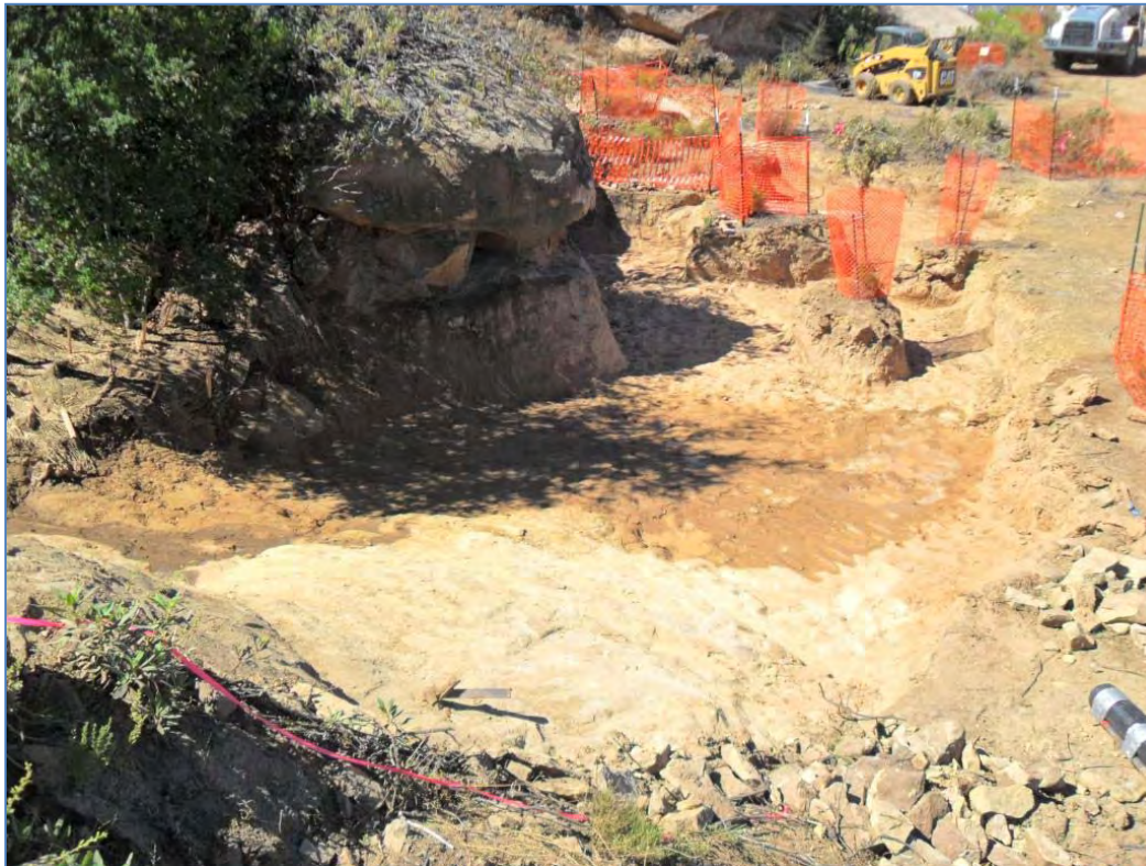
ISRA area B1-1A after excavation (8/23/2010, looking southwest). Bedrock exposed in excavation floor is visible in the foreground. Orange fencing around Santa Susana tar plants.
