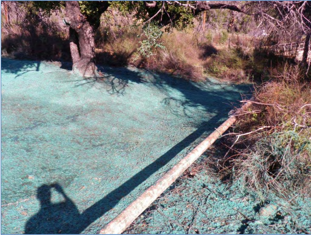
ISRA area AP/STP-1A after restoration (12/3/2010, looking northeast). Blue-green hydroseed mulch is visible.
