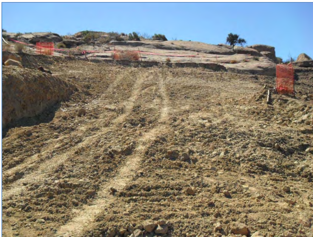
ISRA area B1-1B after excavation (8/23/2010, looking south). Orange fencing around Santa Susana tar plants.
