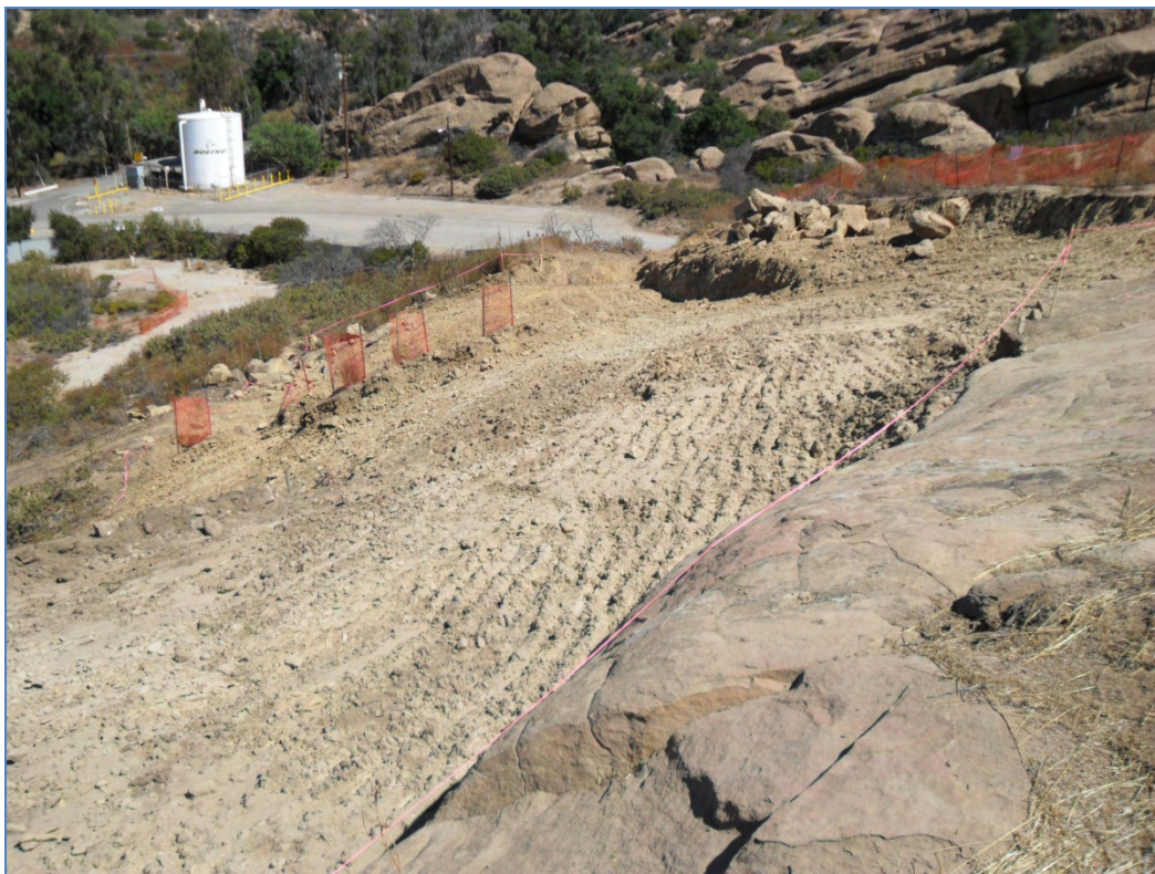
ISRA area B1-1B after excavation (8/23/2010, looking north). Orange fencing around Santa Susana tar plants.
