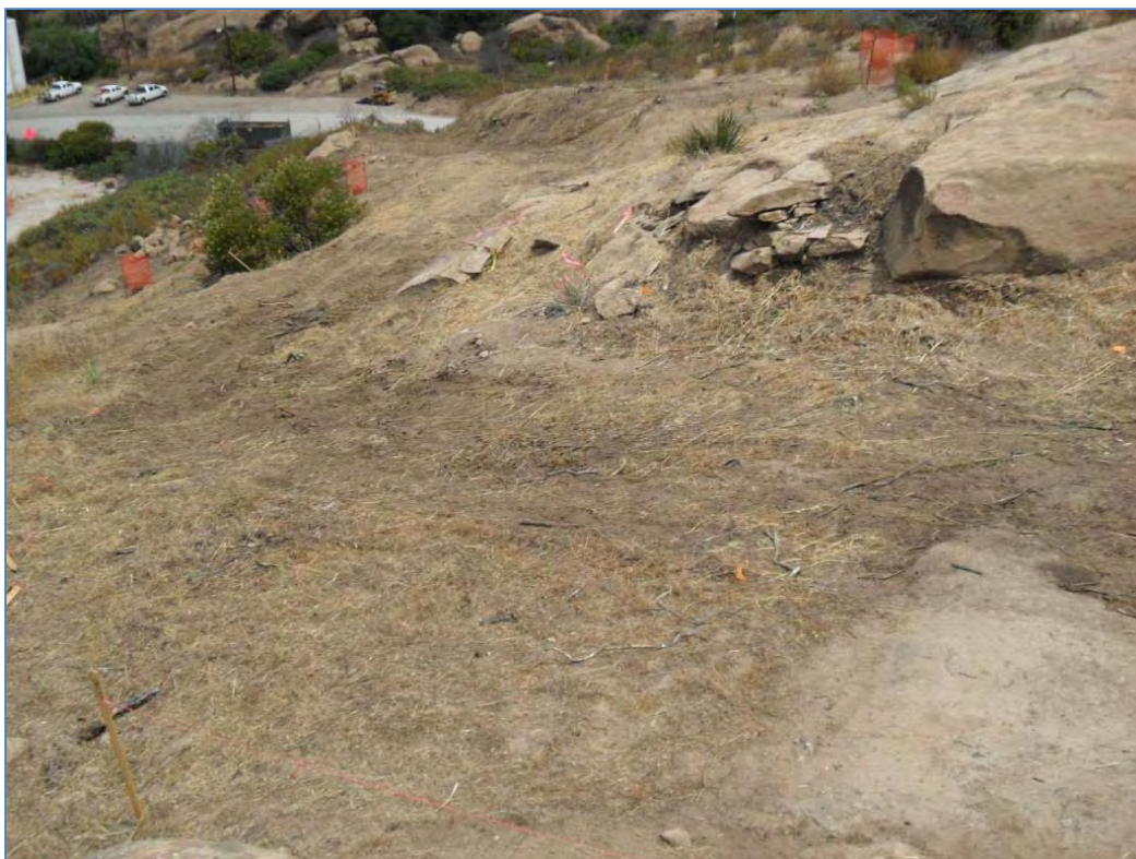
ISRA area B1-1C in foreground and ISRA Area B1-1B in background after vegetation clearance, prior to excavation (7/16/2010, looking north).
