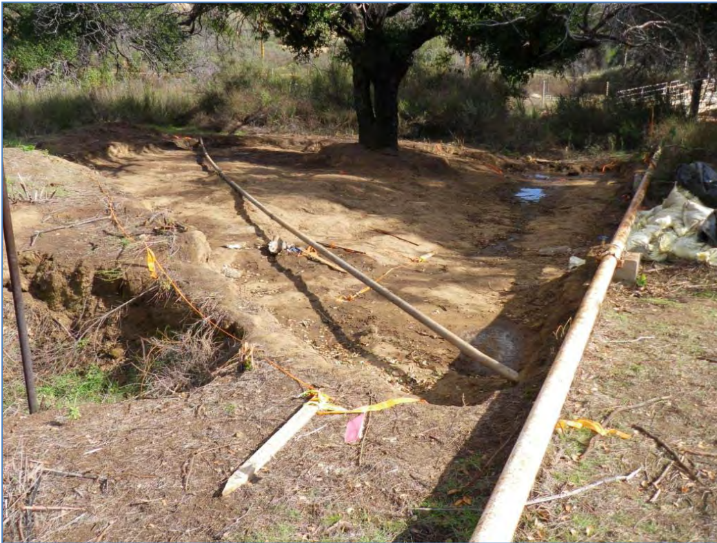
ISRA area AP/STP-1A after excavation (11/23/2010, looking east). The smaller-diameter pipeline through the excavation was subsequently removed (see Appendix H for details).
