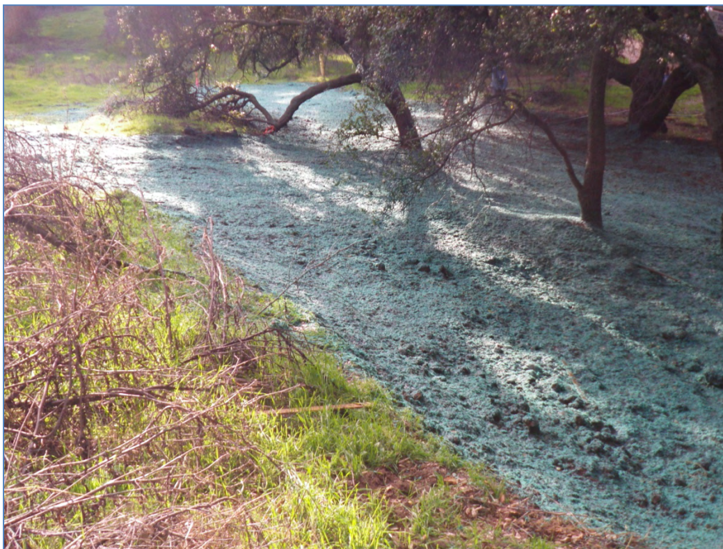
ISRA area AP/STP-1F after restoration (12/2/2010, looking southwest). Blue-green hydroseed mulch is visible.
