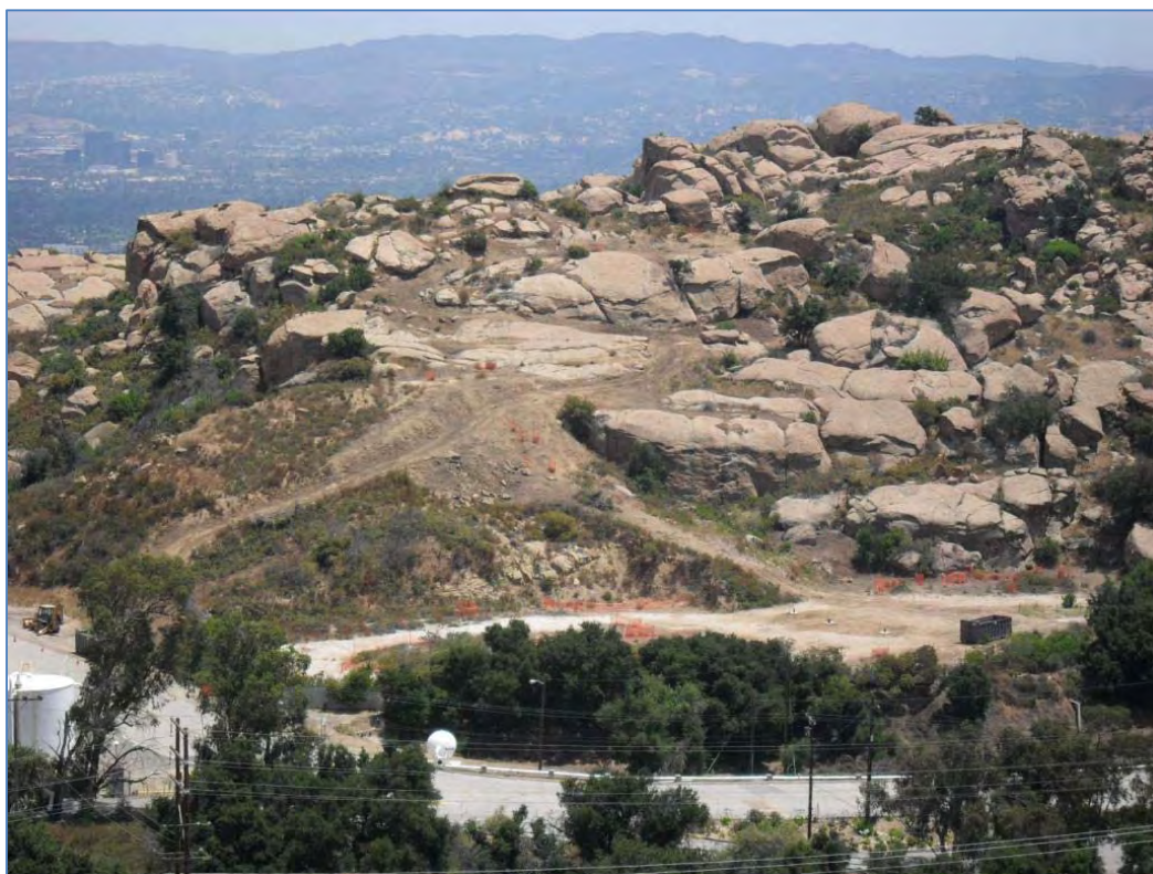
ISRA areas B1-1 and B1-2 after vegetation clearance, prior to excavation (7/16/2010, looking south). Orange fencing around Santa Susana tar plants.
