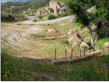
HVS-2A Native plants and additional BMPs installed (looking South). Orange and green pin flags show plant locations. April 2010
