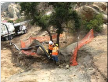
HVS-2A During excavation, vacuuming around oak tree to protect roots (looking Southwest).
