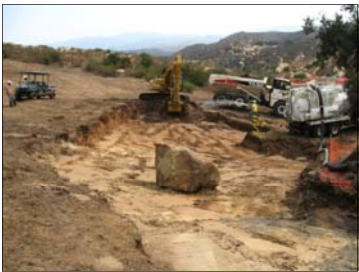
HVS-2A Excavation, and conditioning soils using water spray for dust control (looking South).
