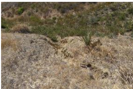
Picture #32: Looking east at rill on south/southeast side of road.
