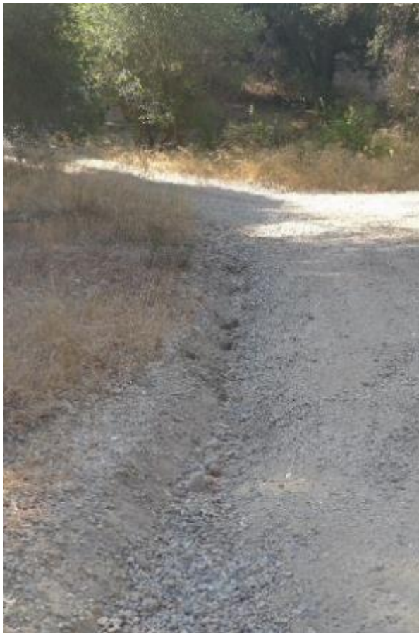
Picture #28: Looking southeast at erosion along northeast side of road.
