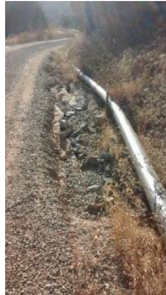
Picture #2: Looking southeast at rill near culvert.
