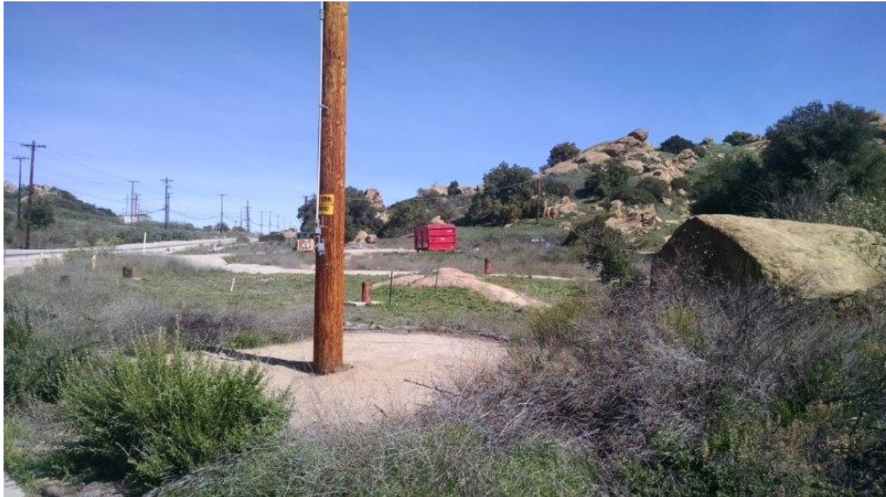
Figure 3. Example of new treated wood pole, EPTWBS03.
