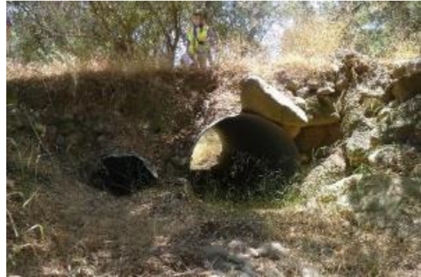
Picture #27: Looking south at culverts under road. Culvert on the left is partially blocked.
