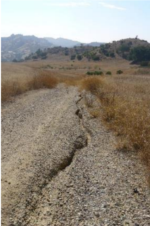
Picture #35: Looking southeast at rill development along south side of road.
