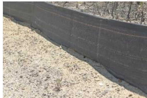
Picture #19: Looking south at loose silt accumulating along silt fence.
