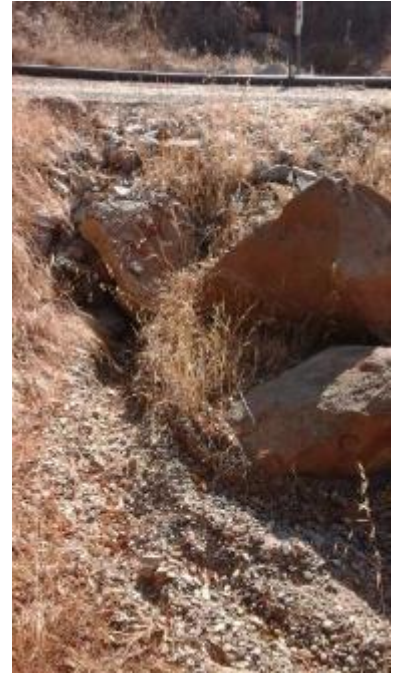
Picture #12: Looking east at erosion upgradient of culvert pipe.
