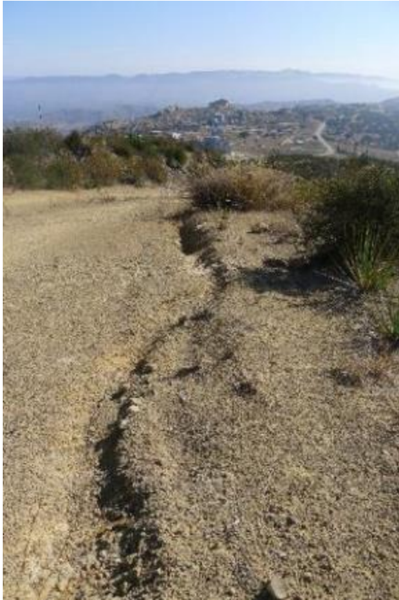
Picture #34: Looking northeast at rutting along southwestern side of road
