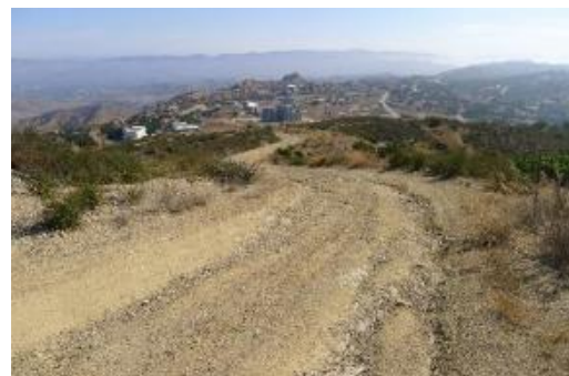
Picture #33: Looking northeast at rutting across road.
