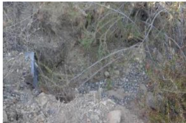
Picture #4: Looking northwest at northern side of culvert where gravel from the road has been deposited in the drainage.
