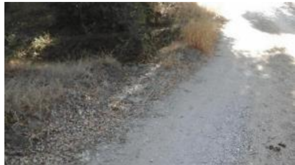
Picture #29: Looking east at erosion at northwest corner of culvert crossing.
