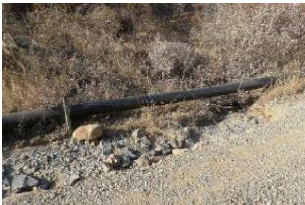
Picture #3: Looking southwest at rill underneath HDPE pipe near culvert.
