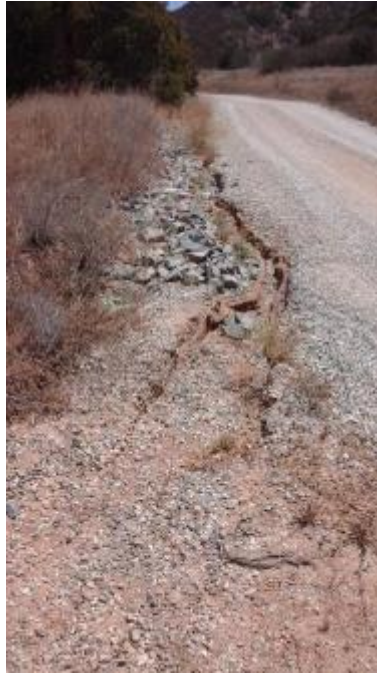
Picture #24: Looking southeast at erosion along north side of road.
