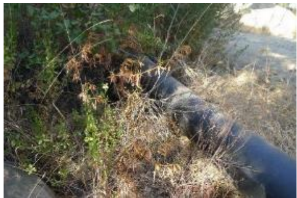
Picture #6: Looking southwest at erosion underneath HDPE pipe
