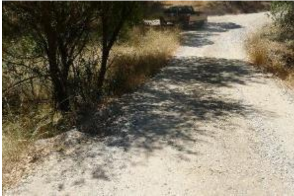
Picture #26: Looking west at erosion on southeast corner of culvert crossing.
