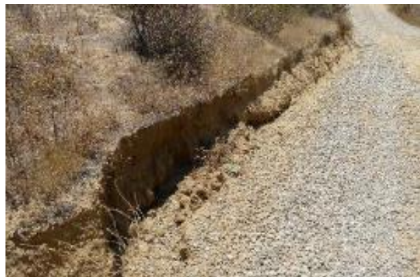
Picture #21: Looking southwest at slope failure along south side of road.
