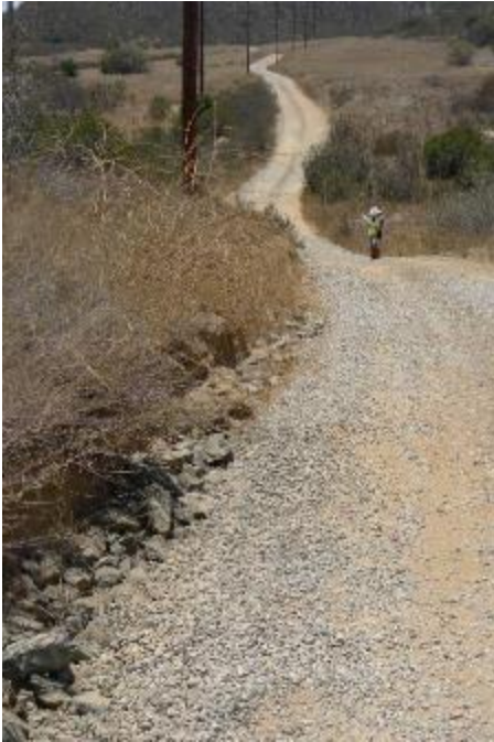
Picture #22: Looking southwest at rip rap and erosion on south side of road.
