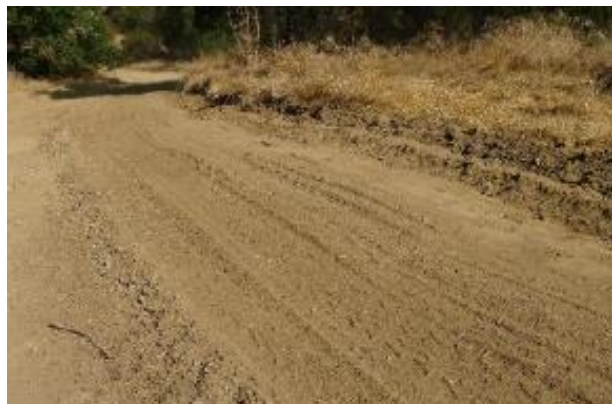
Picture #31: Looking east at fine sediment on road surface.
