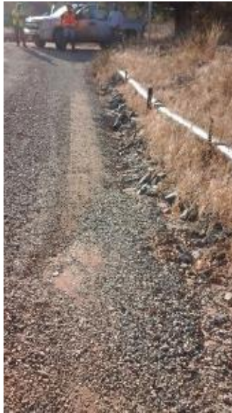
Picture #1: Looking southeast at rill near locked gate #575.
