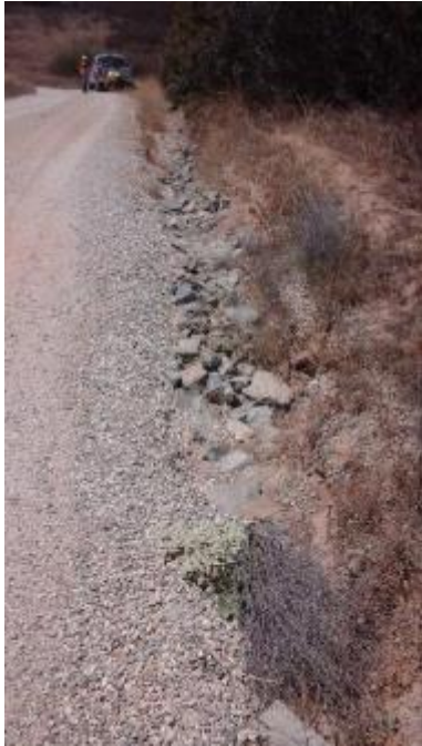
Picture #23: Looking northwest at erosion along north side of road.
