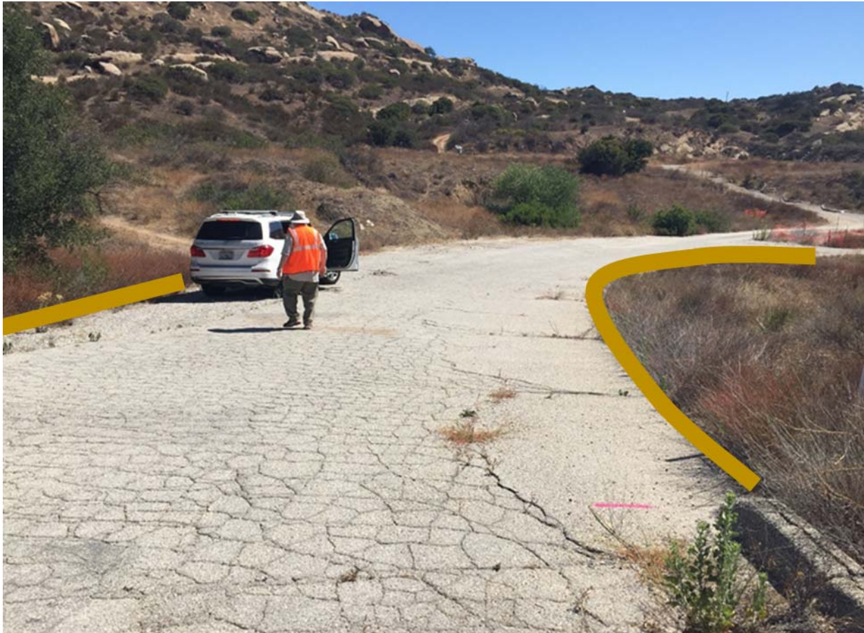
Figure 19. Proposed Location of Sand Bags to Divert Stormwater to Adjacent Vegetated Areas
